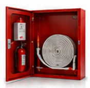
Fire Hose Cabinet
